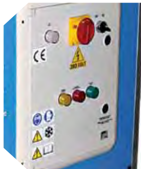
Detail of the control lights of the h.p. line
